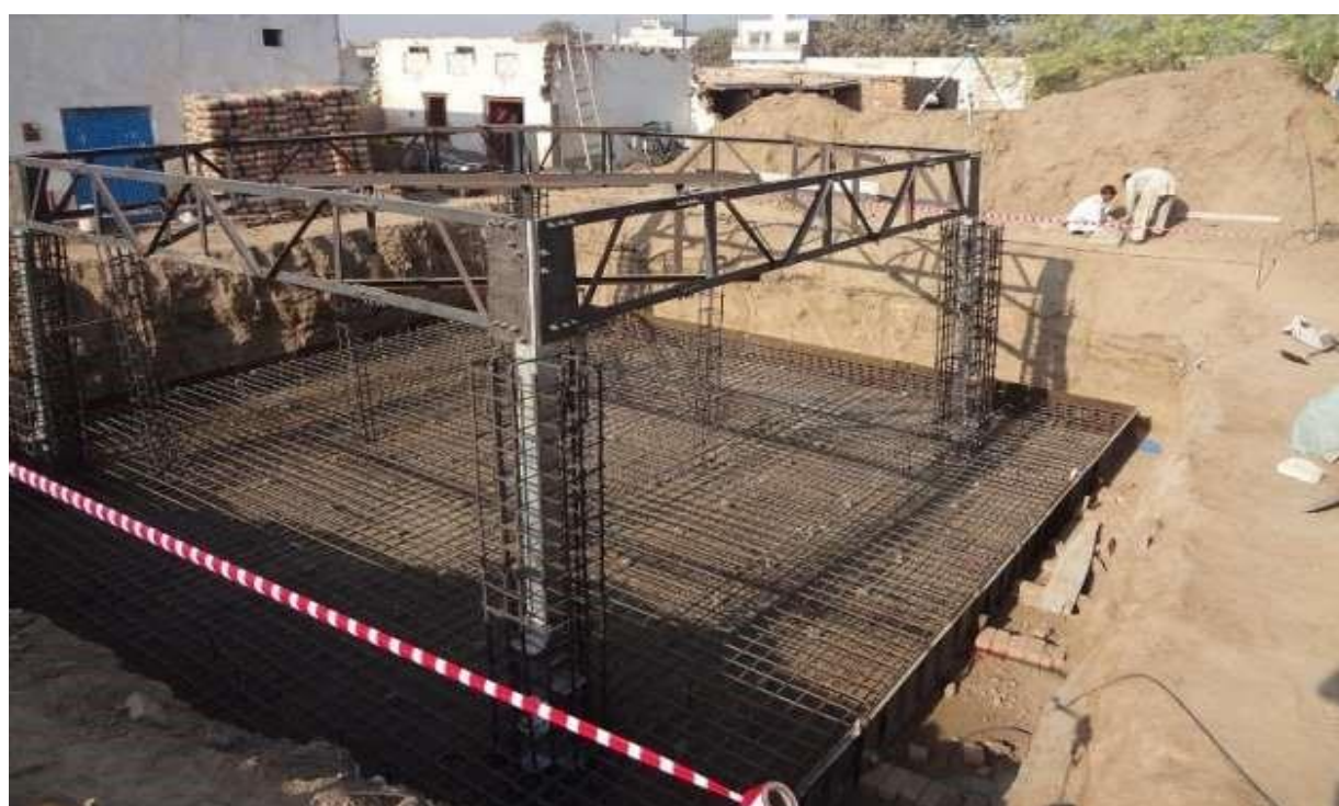
130-MUL-0227 Multan City, Mobilink C-III, BTS Site 46 M
